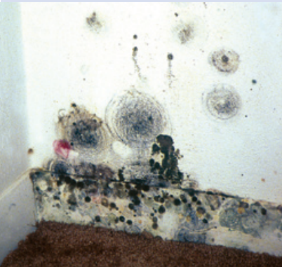
Photo 3A: Mold growing in closet as a result of condensation from room air
