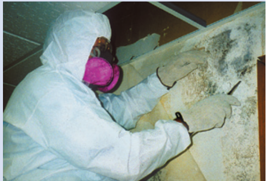
Photo 7: Remediation worker with limited PPE
