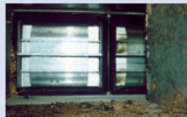
Photo 4C: Moldy air duct
