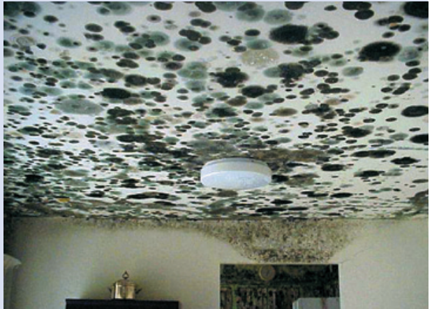
Photo 2: Extensive mold contamination of ceiling and walls
