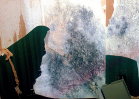
Photo 5: Mold growth behind wallpaper
